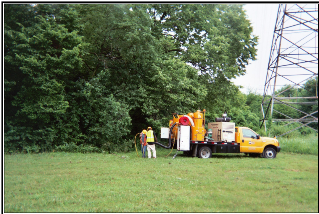
Figure 4.3. Example of a crew vacuuming the top 1.8 to 2.4 m (6 to 8 ft) of soil at bore hole 3B-197.
