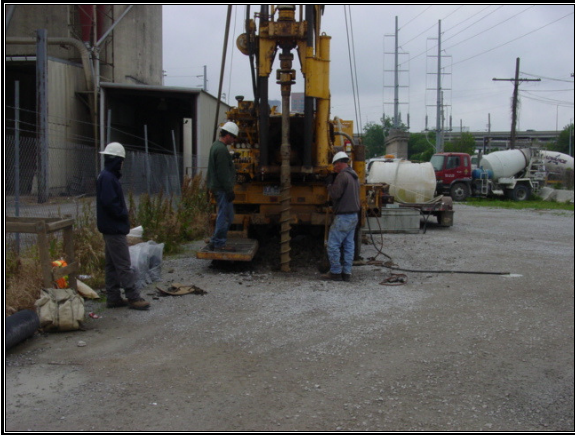
Figure 6.30. Overview of bore holes in Locality 16 at the concrete plant, looking northeast.
